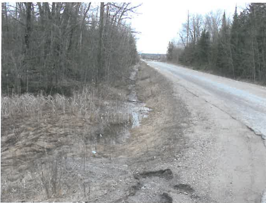
Photo 19 - Campbell Drive Roadside Ditch looking south from the "T" intersection with Usborne Street.
