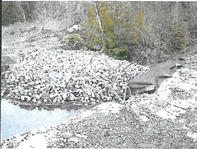
Photo 3 - RipRap Check Dam at Sediment Basin Outlet
