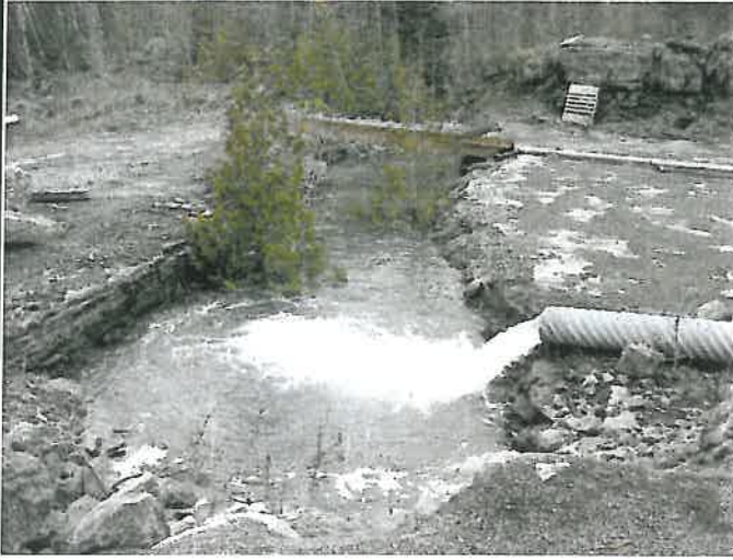
Photo 2 - Pump Discharge to Sediment Basin
