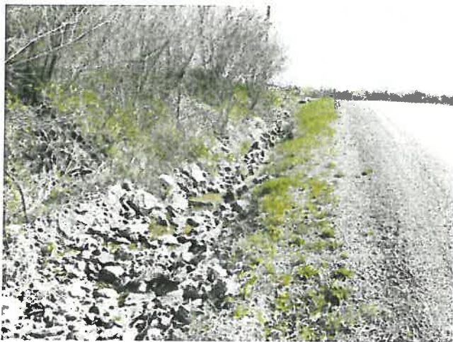
Photo 1: SW 5, looking north-east along Carmichael Side Road. Campbell Road is at top of road (see Culvert), May 9, 2011
