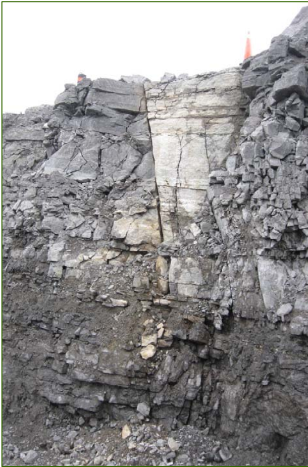
Photo 6: Joints, enhanced in weathered bedrock zone, extend down to the contact between Bobcaygeon and Gull River Formations (November 23 2009 photo)
