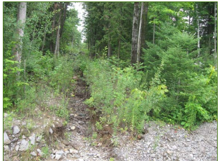
Photo 11: Portion of Ditch constructed to Divert Seasonal Springwater Flow in the Subdivision (July 24 2009 photo)
