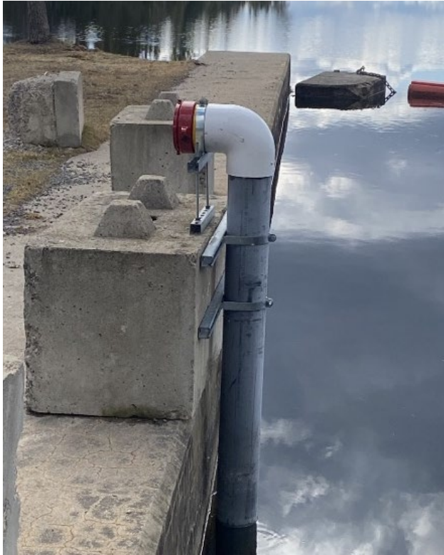
Figure 10. Dry hydrant installed at White Lake.
